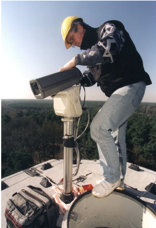
Abbildung 5.8: Installation eines Systems FIREWATCH in Brandenburg.
