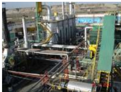
Industrial installation, Peru (Photo: CENACID)
